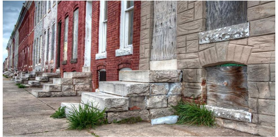
Marble stairs showing signs of weathering in Baltimore City, MD.
