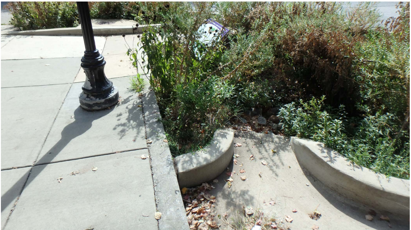
Inlet and vegetation in curb bump-out, Baltimore, MD.
