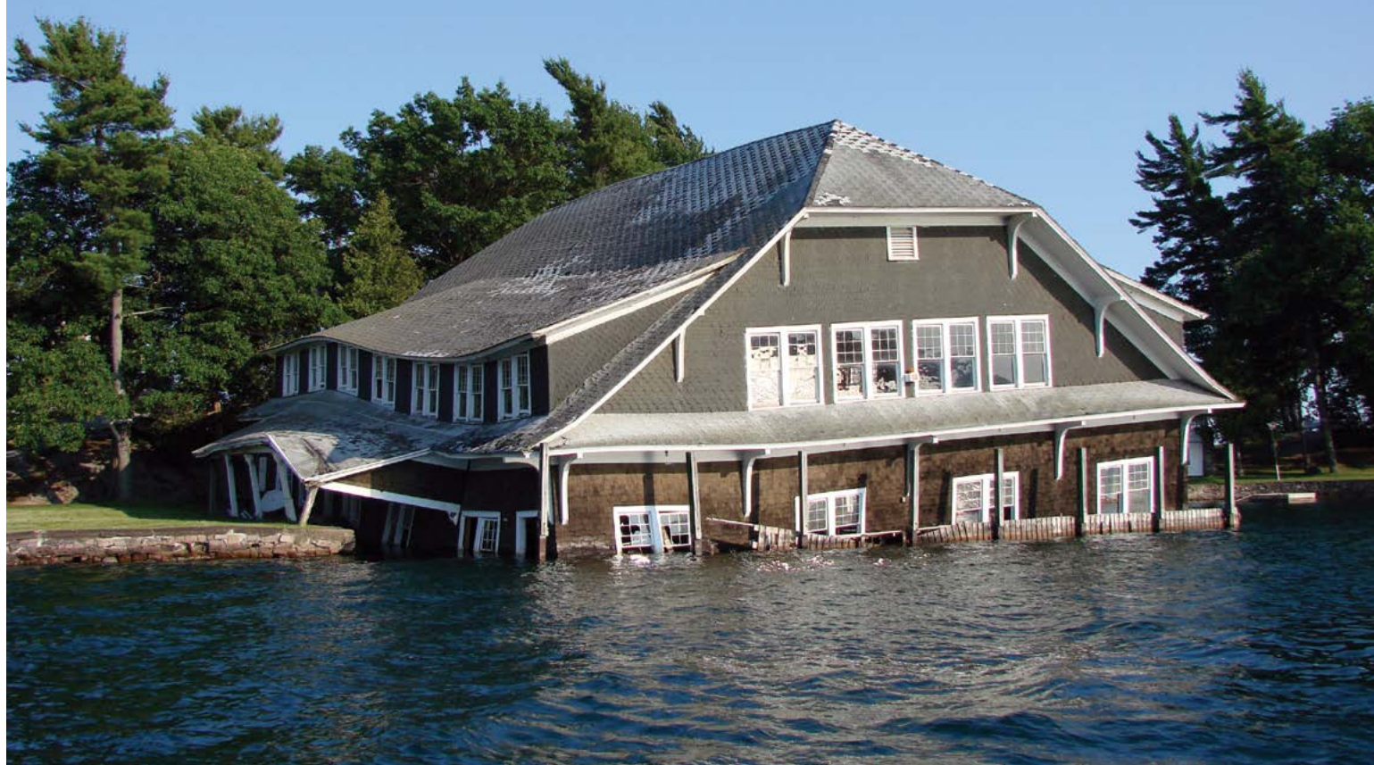
Building too close to the shore often removes stabilizing vegetated buffers and leaves properties vulnerable to erosion and flooding damage.
