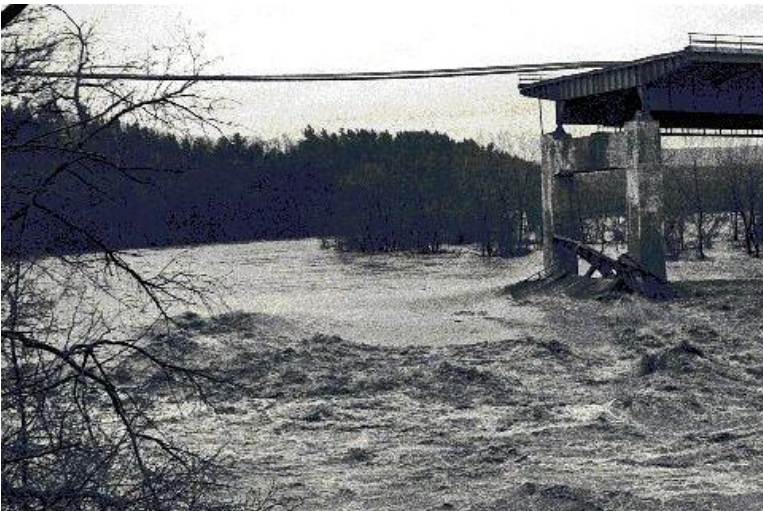
The remains of the I-90 (New York State Thruway) bridge over Schoharie Creek, New York, after a flood undercut the bridge supports and destroyed the bridge. Credit: USGS - http://water.usgs.gov/wid/images/NY.figure.id.3.gif , Public Domain, https://commons.wikimedia.org/w/index.php?curid=56907491
