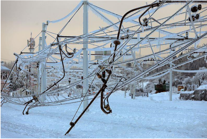
Damage from freezing rain. Credit: Wikipedia.
